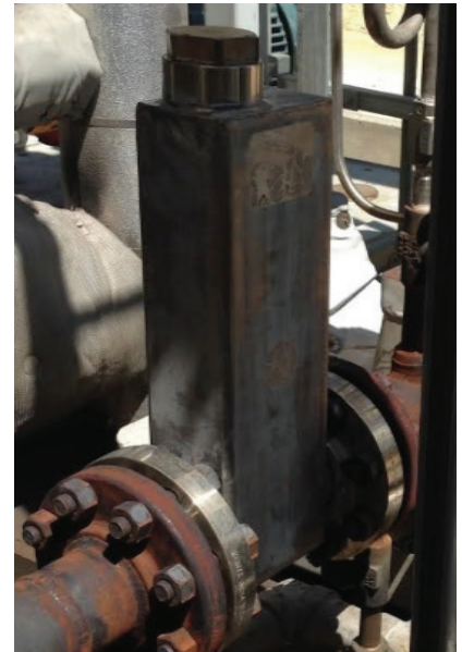
Figure 1. Black Powder Solutions Magnetic Separator installed upstream of the pump
