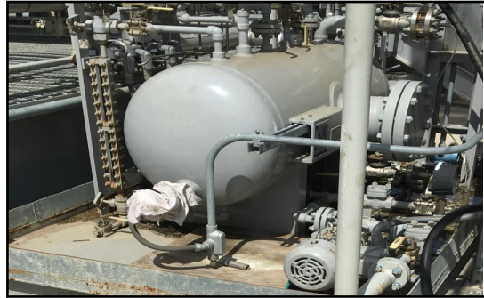
Reclaimed oil tank.
